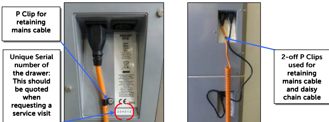
Figure 1: Mains Connection Point
